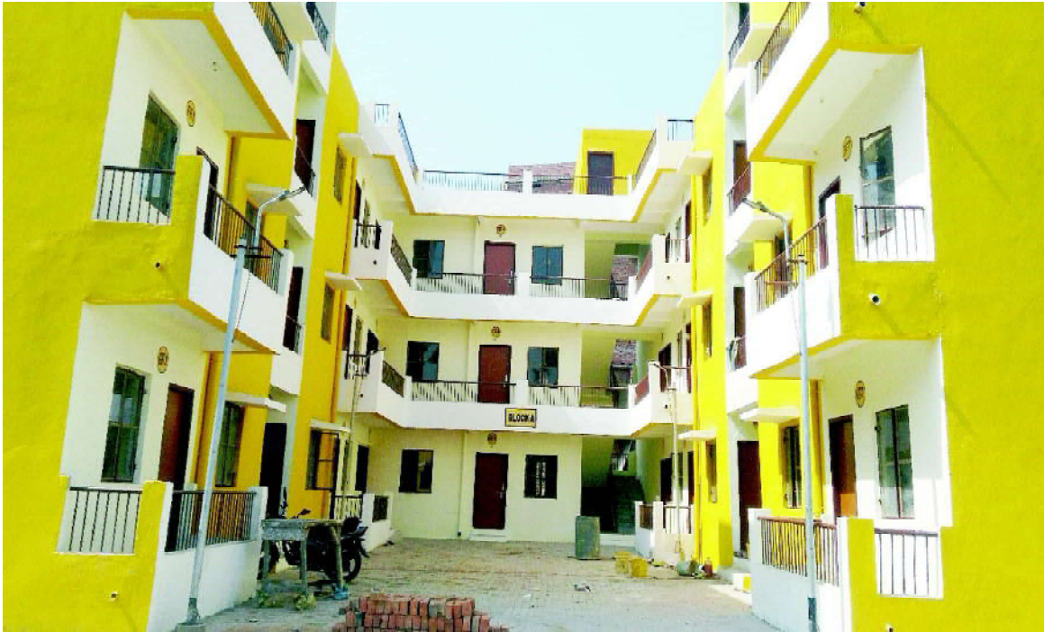
Demonstration Houses (36 DUs) being constructed using Coffers Structural Stay in Place Formwork System by BMTPC at Bihar Shariff, Bihar
