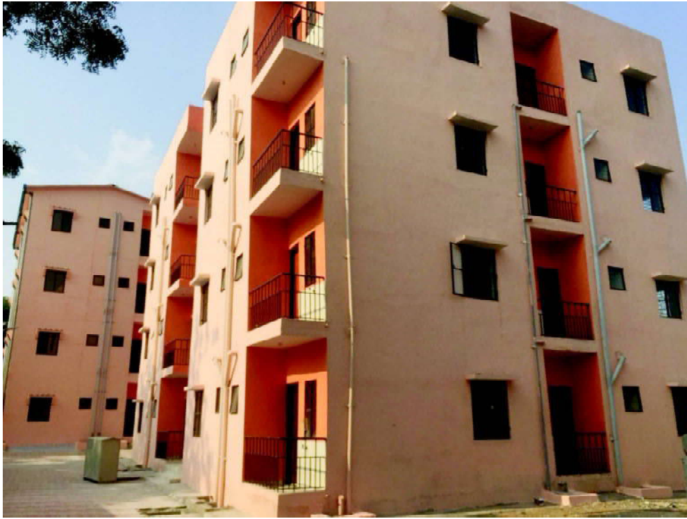
Demonstration Houses constructed using Coffor Structural Stay in Place Formwork System (16 houses) and Light Gauge Steel Frame System (16 houses) by BMTPC at Gachibowli, Hyderabad, Telangana
